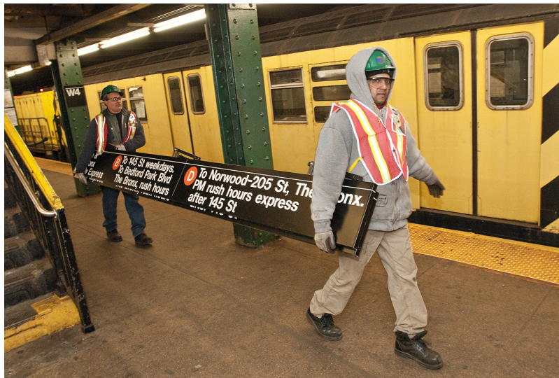
Figure 11.3.1: The New York City Metropolitan Transit Authority undertook a new approach to how they perform critical inspection and maintenance of subway components that are necessary to providing reliable service. Rather than schedule these inspections during regular hours, they consulted with the maintenance workers, who suggested doing the inspections while sections of the subway were closed to trains for seven consecutive hours. This process was adopted and provided a safer and more efficient way to maintain and clean New York City's sprawling subway. With no trains running, MTA employees are able to inspect signals, replace rails and crossties, scrape track floors, clean stations, and paint areas that are not reachable during normal train operation. Workers also took the opportunity to clean lighting fixtures, change bulbs, and repair platform edges while performing high-intensity station cleaning. (Credit: Patrick Cashin/ flickr/ Attribution 2.0 Generic (CC BY 2.0))
