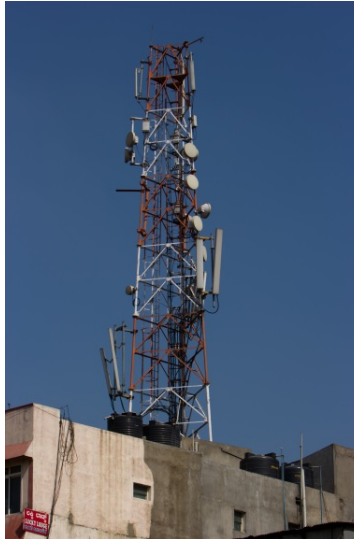
Figure 9.13.1: India has the world’s second-largest mobile-phone user base: 996.66 million users as of September 2015. Shown here is a rooftop mobile phone tower in Bangalore.
