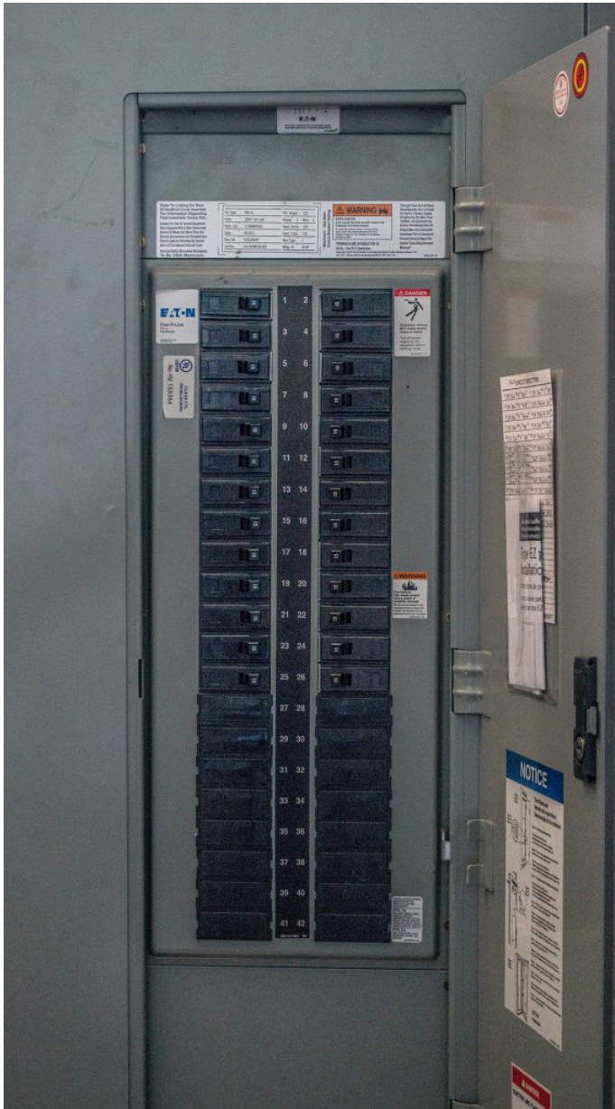
Panelboard by Gwen Arkin is licensed under CC BY 4.0
