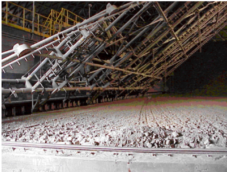
Figure 4.2.4.32: Raking device for reclaiming stored limestone (Copyright Halliburton Energy Services).
