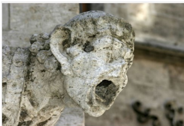
Figure 7.6.3. A gargoyle that has been damaged by acid rain.
