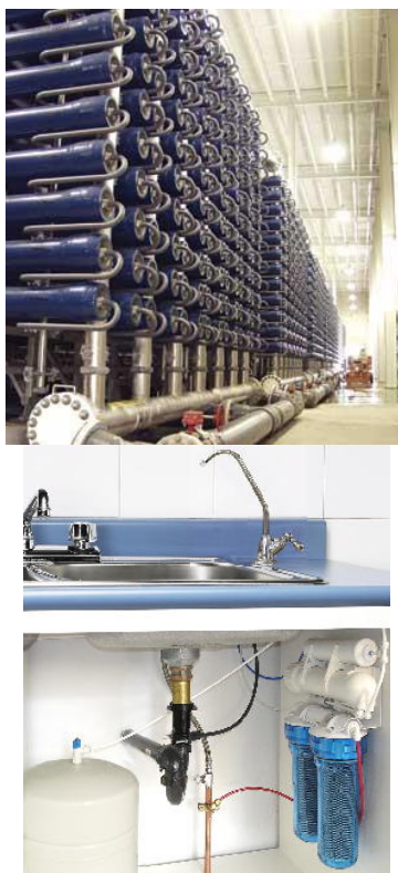
(left) Large-scale RO plants use multiple membrane cartridges. This one, in Tampa Bay FL, supplies desalinated drinking water to 2.4 million residents. (right) Many smaller RO units, suitable for home use, can fit under a kitchen sink.
