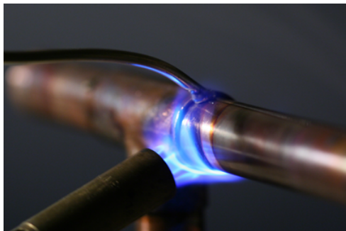
Figure 4.3.4: Propane torch being used to solder copper pipes for residential water mains. Source: Kevin L Neff / CC BY ( https://creativecommons.org/licenses/by/2.0 )
