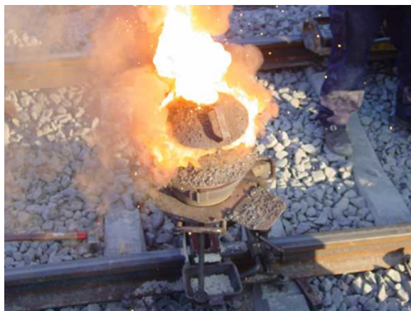
Figure 4.3.1: Thermite reaction proceeding. Shortly after this, the liquid iron flows into the mold around the rail gap. Source: http://en.Wikipedia.org/wiki/Image:V...ewelding-1.jpg , Public domain.
