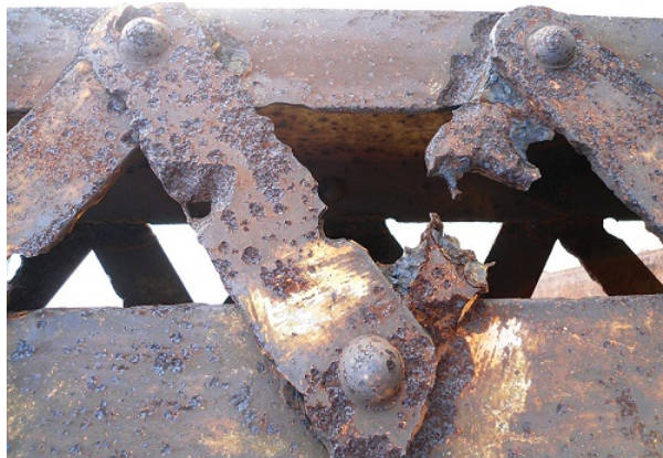
Figure 15.1.1: Corroded beams on the Nandu River Iron Bridge. These support beams on the bridge are obviously rusted. If the rusting becomes too bad, it will compromise the integrity of the bridge, requiring replacement. (Public Domain; Anna Frodesiak.)
