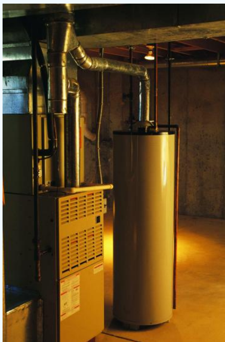
Figure 11.3.2 Tank water heater © Thinkstock. Most homes in the United States have a tank-type water heater like this one.
