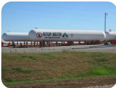
Figure 19.8.1: An ammonia storage tank.
