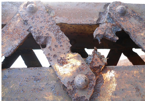
Figure 14.1.1: Corroded beams on the Nandu River Iron Bridge. These support beams on the bridge are obviously rusted. If the rusting becomes too bad, it will compromise the integrity of the bridge, requiring replacement. (Public Domain; Anna Frodesiak.)
