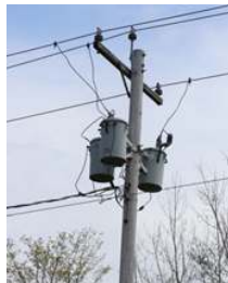
Figure 10.4.2 : A cluster of three residential power transformers.
