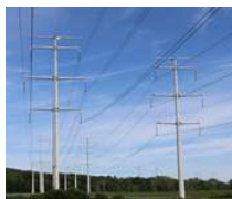
Figure 1.1.1 : 345,000 volt transmission lines.
