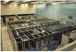
The CERN data center in 2010 housing some WWW servers
